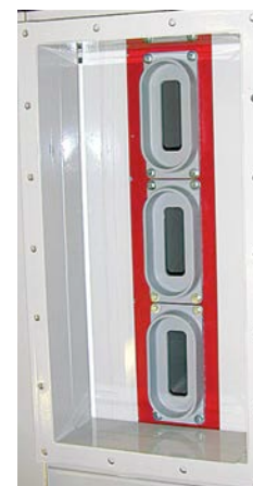
Vertical bus supports
