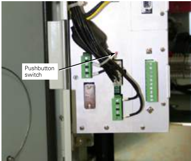
Figure 39. Location of pushbutton switch on the SPEAR single-phase recloser control side-panel for power-up with battery power only
