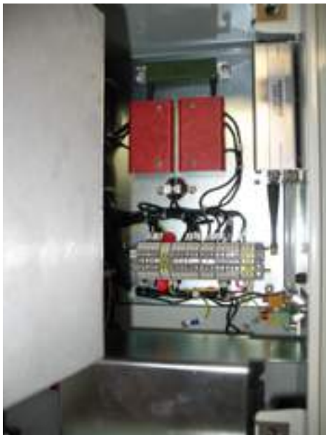
Figure 26. Radio mounting tray (example radio mounted) mounted on right-side interior cabinet wall
