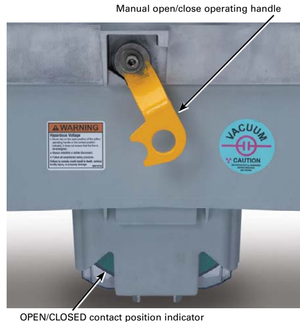
Figure 10. NOVA NX-STS recloser operating handles and position indicators
