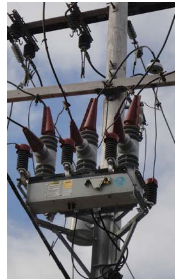
Three-phase NOVA recloser on one end of an AST application.
