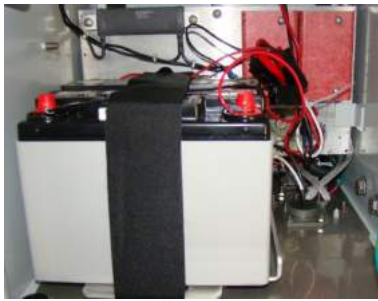
Figure 1. 24 Volt DC 13 Ahr battery strapping
