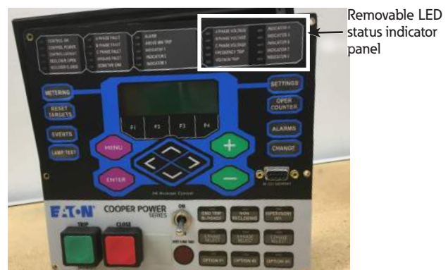
Figure 27. Open front panel. Labels are easily removed from and inserted into the top of the programming panel LED status indicator section
