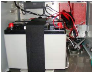
Figure 1. 24 Volt DC 13 Ahr battery strapping
