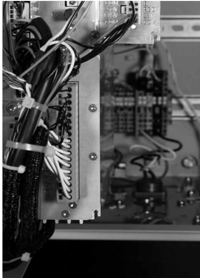
Figure 19. Contact I/O Module
