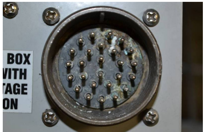
Figure 3. Corrosion residue left on 26-pin J-Box receptacle
