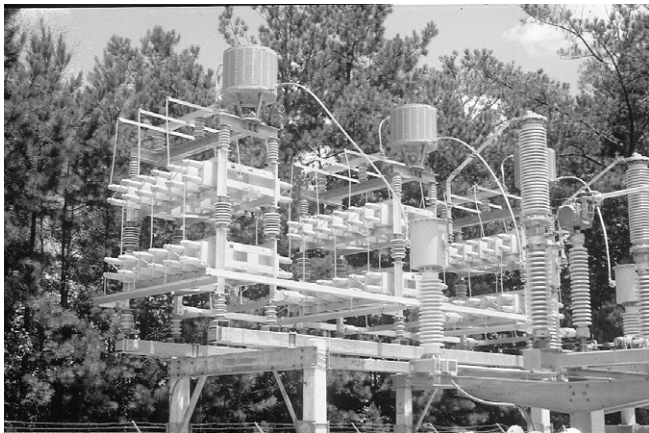
Figure 1. Fuseless capacitor bank
