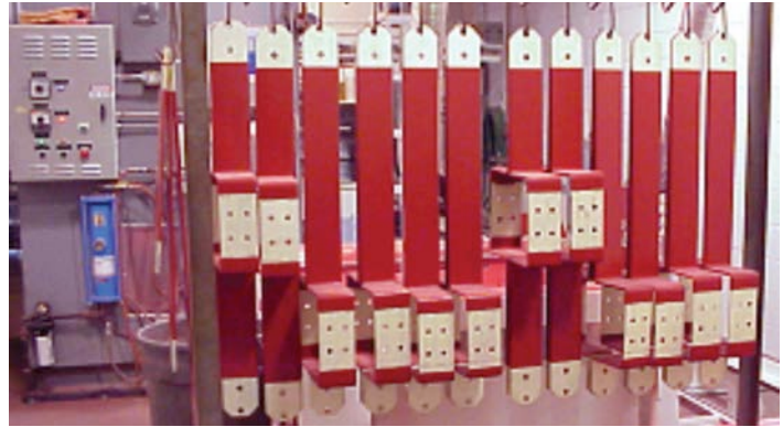
Fully silver-plated copper bars with red epoxy insulation
