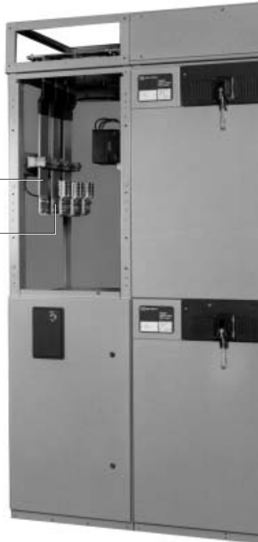
Typical 26-Inch (660.4 mm) Wide Incoming Line Structure
