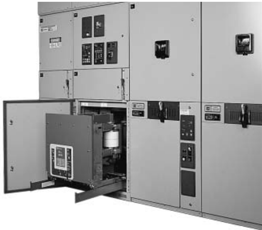
Main Breaker Ampgard — Breaker Withdrawn
