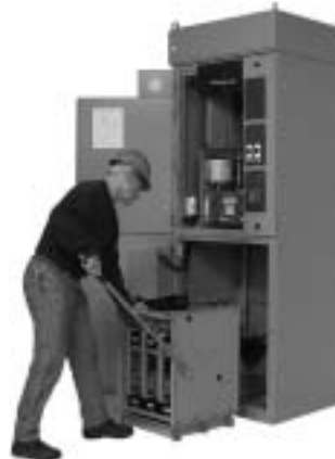
SCR Truck Removal
