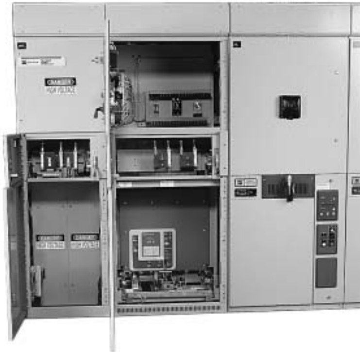
Main Breaker Ampgard — Breaker Connected
