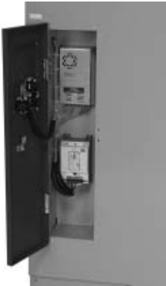
Lower Compartment Low Voltage Door
