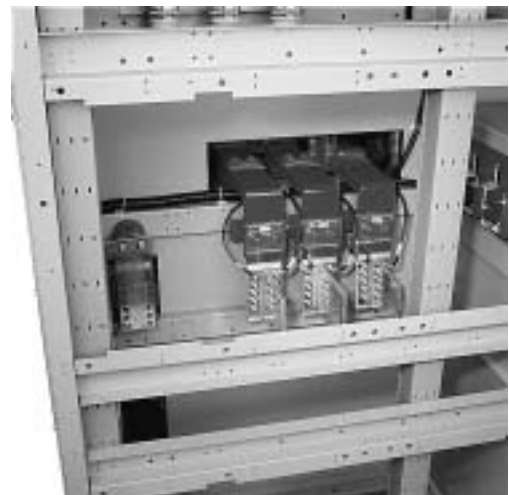
Side Panel Removed to Show Incoming Cable Connections
