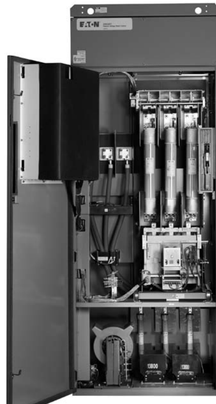
15 kV AMPGARD Starter—Medium Voltage Door Open
