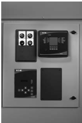
Low Voltage Door with InsulGard Relay
