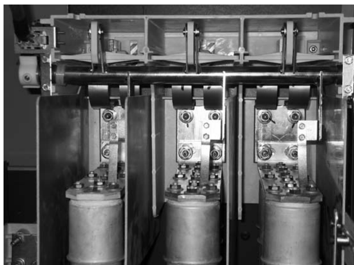
View of Isolation Switch Through Viewing Window
