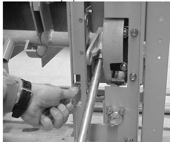
Fig. 8 Override of Switch Interlock Safety Latch
