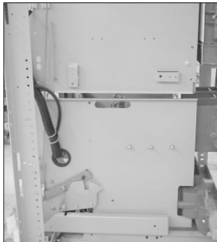
Fig. 9 Contactor Open, Interlock Neutral
