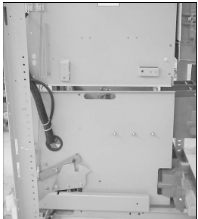
Fig. 8 Contactor Open, Interlock Neutral
