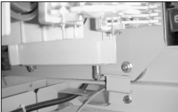
Fig. 12 Code plate in 400 amp cell preventing 200 amp contactor from being inserted.
