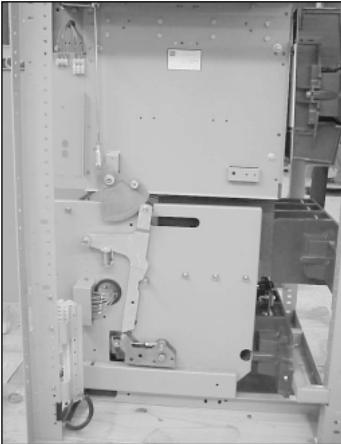
Fig. 14 Contactor Interlocked Open by Isolation Switch
