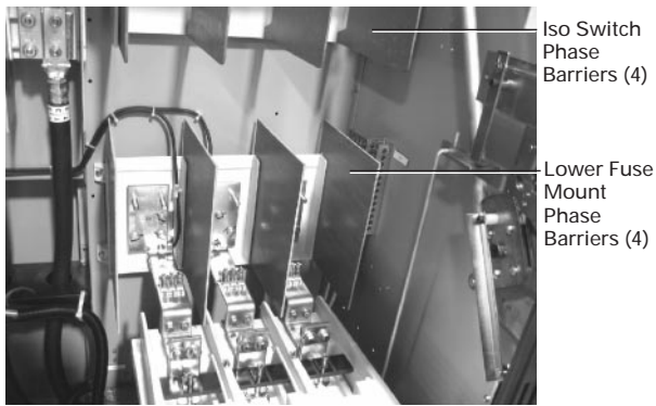
FIGURE 18. LOWER FUSE MOUNTING WITH PHASE BARRIERS INSTALLED
