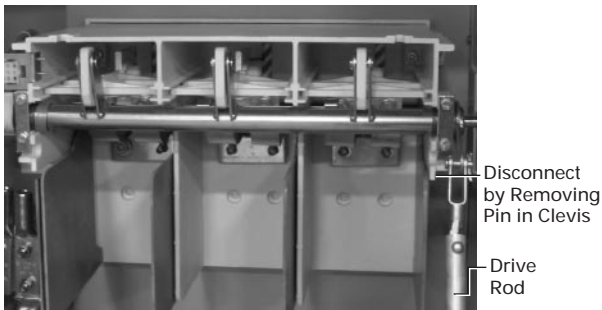
FIGURE 26. ISOLATION SWITCH DRIVE ROD
