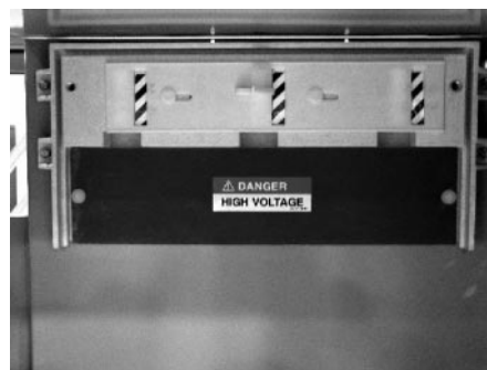
FIGURE 5. FIXED PORTION — ISO SWITCH
