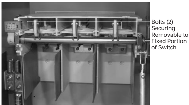
FIGURE 27. BOLTS SECURING ISOLATION SWITCH
