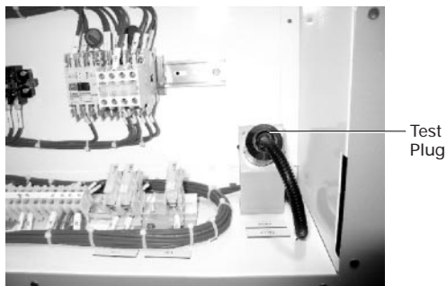
FIGURE 11. LV COMPARTMENT WITH TEST PLUG
