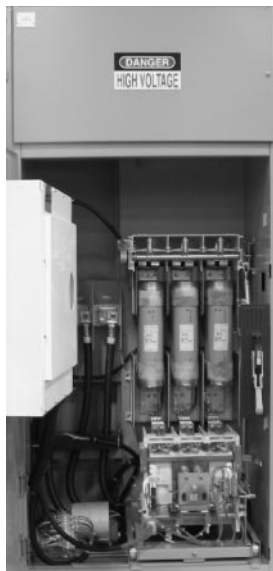
FIGURE 2. MEDIUM VOLTAGE COMPARTMENT
