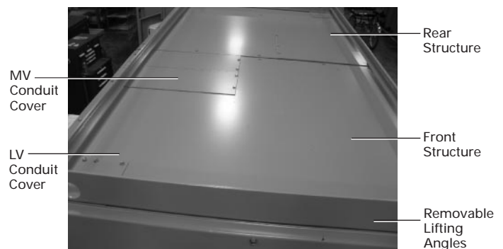
FIGURE 15. TOP COVER (VIEW FROM FRONT OF BUS COMPARTMENT, BACK-TO-BACK STRUCTURES)
