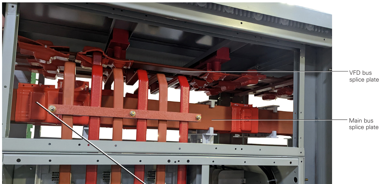
Access to the bus compartment from rear side to connect the busbars with splice plates.
