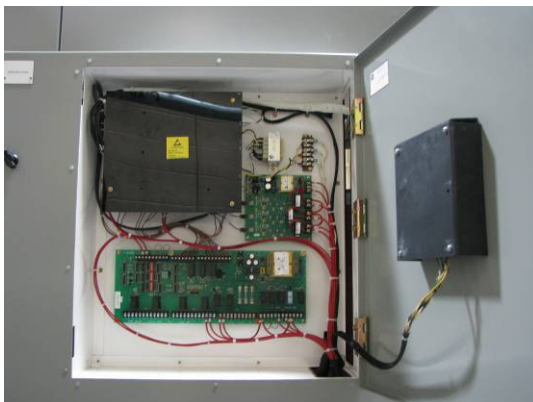
Figure 8. Control System Boards
