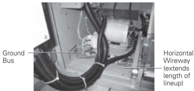
Figure 18. Horizontal Wireway and Ground Bus
