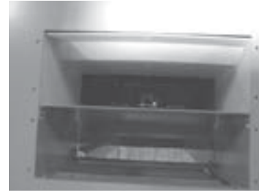
Figure 16. Medium Voltage Cable Conduit Area (View from Top Rear of Bus Compartment)
