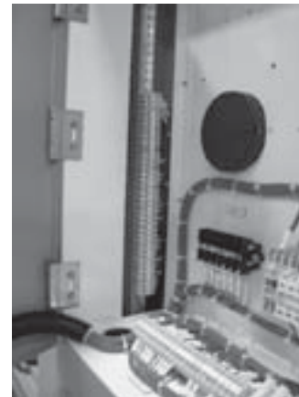
Figure 10. Low Voltage Terminal Blocks, Low Voltage Door Open
