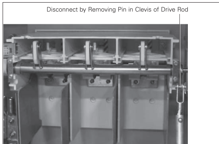
Figure 31. Isolation Switch Drive Rod
