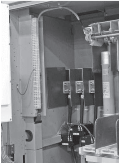
Figure 11. LV Terminal Blocks, MV Door Open
