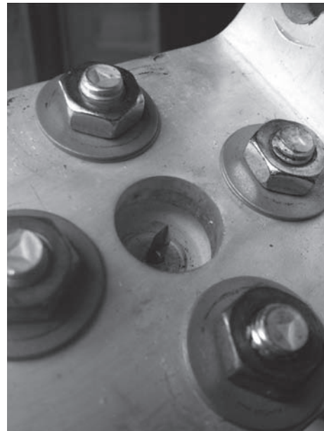
Figure 8. Blown Fuse Indicator
