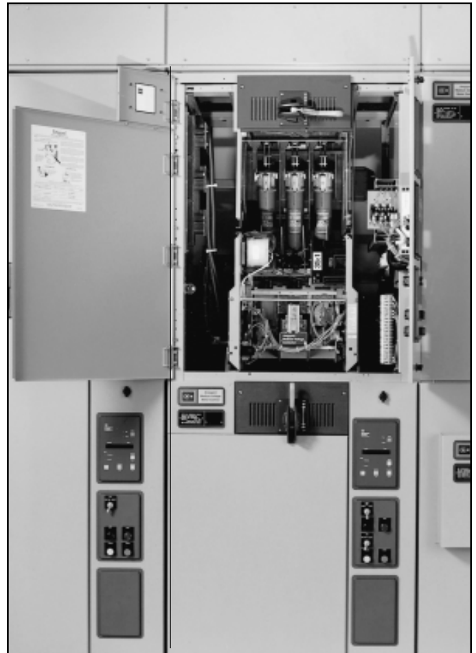
Fig. 14 Controller With Doors Open
