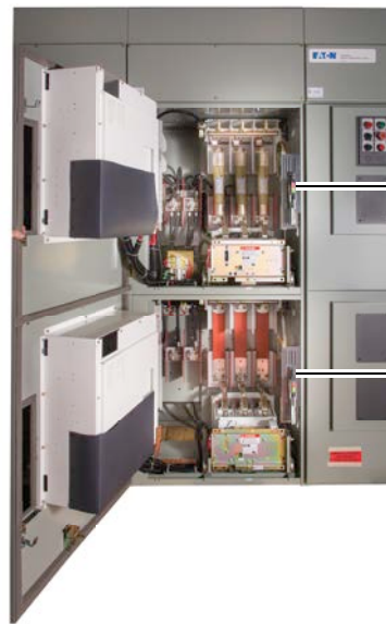
400 A motor bypass starter and motor select contactor assembly
