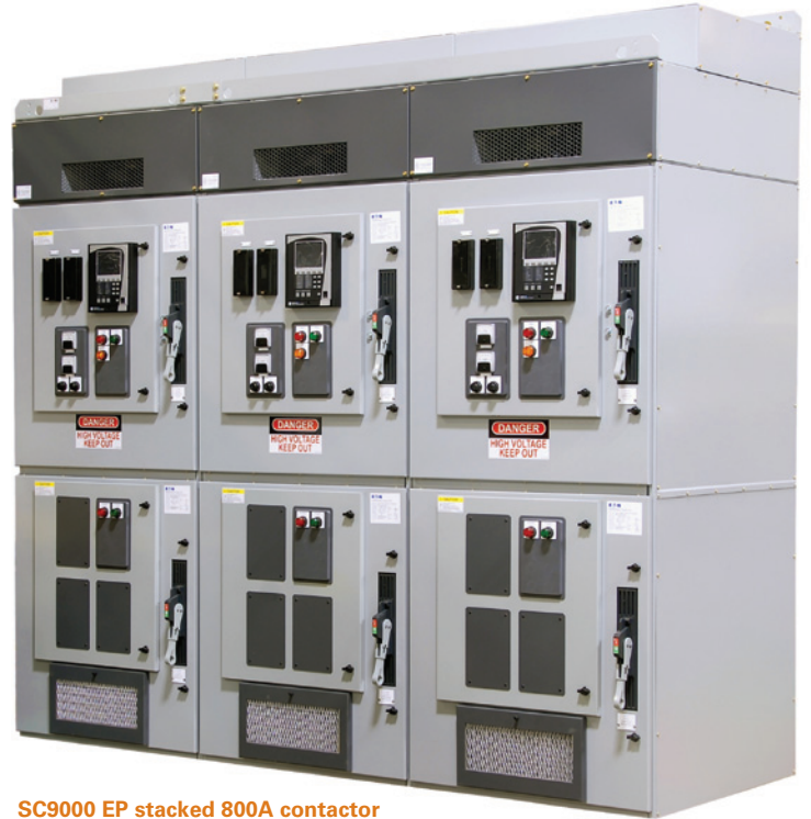
SC9000 EP stacked 800A contactor Closed-transition with stacked 800A contactors
