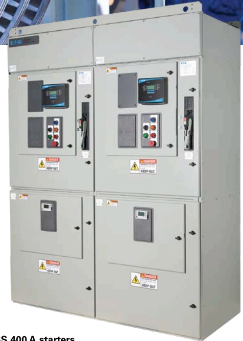
Ampgard RVSS 400 A starters with EMR-4000 relays
