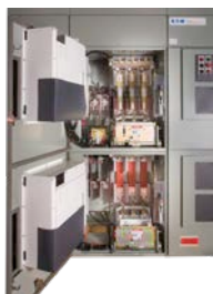
Synchronous transfer with medium-voltage drive
