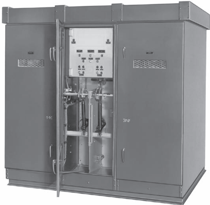
Two-switch automatic transfer
