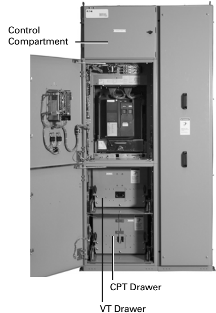
MEF Switchgear—Indoor Unit
