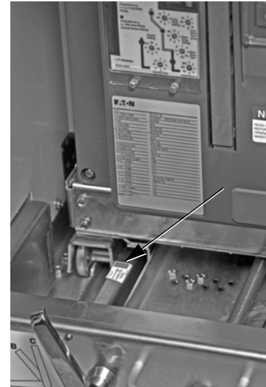
Circuit Breaker in Connected Position Indicator
