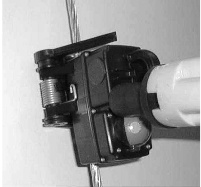
Figure 11. Reset FISHEYE display by touching the reset tool to the FCI housing below and to the left of the pulling eye
