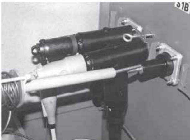
Figure 12. Test for voltage with volt meter
