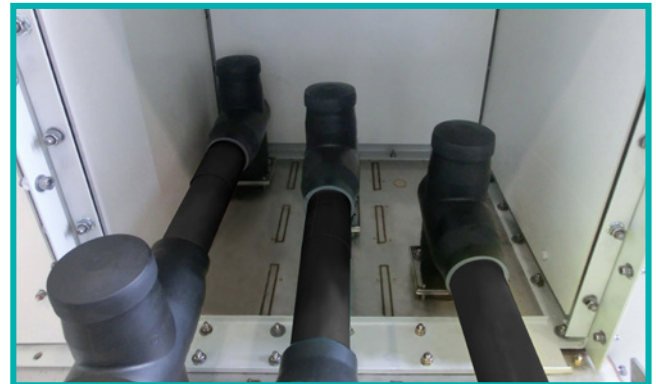
Solid shielded insulation system provides enhanced arc flash safety.
