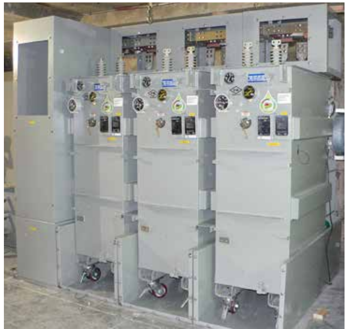
Eaton's Cooper Power series Triplex Indoor-Powercenter tested at 50.6dB (ONAN)/57.8dB (ONAF) - On-site assembly.
