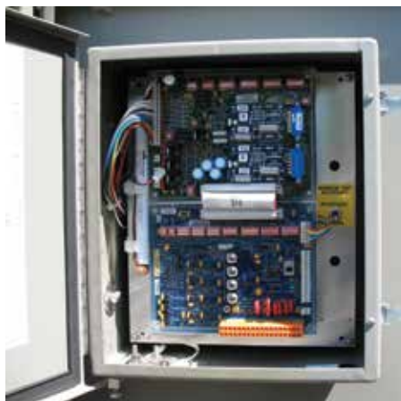
Figure 16. TPG control with SCADA shown.
