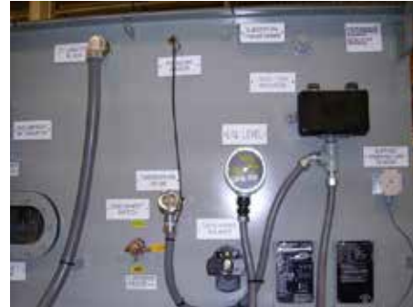
Figure 10. Automation solutions for remote monitoring.
