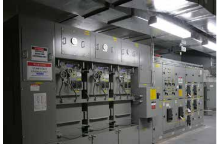
Figure 22. Triplex Indoor Power Center comprised of energy efficient and low noise single-phase substation transformers in a ganged setup.
