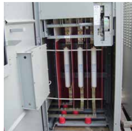
Figure 19. LIS—interior view showing power fuses.
