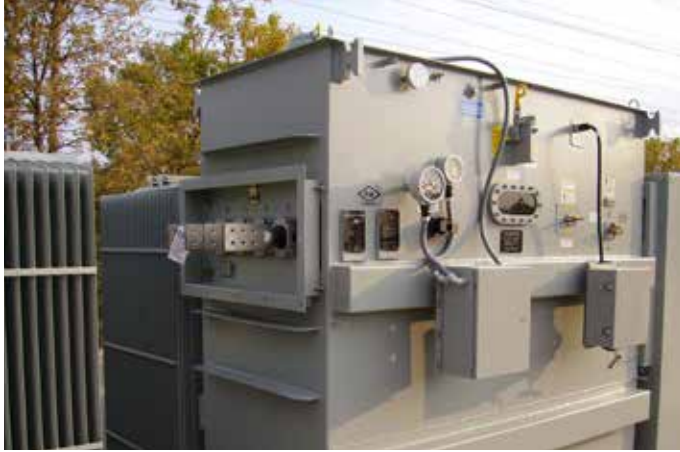
Figure 20. Substation transformer with visible break technology.
