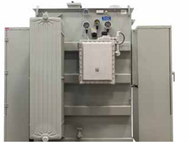
Figure 23. Class I Div 2 hazardous duty substation transformer.
