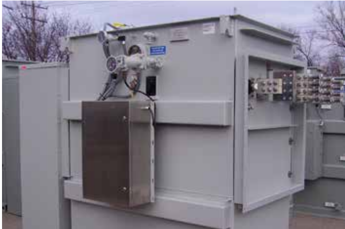
Figure 21. Substation transformer with customer-specific coordination and accessories.
