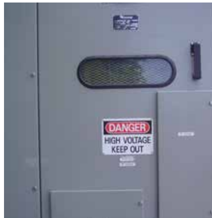
Figure 18. LIS—switch position viewing window.
