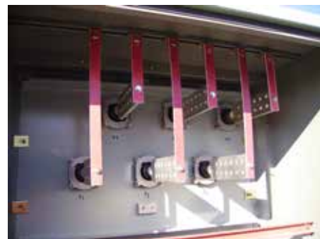
Figure 11. 12-pulse application with bushing supports.
