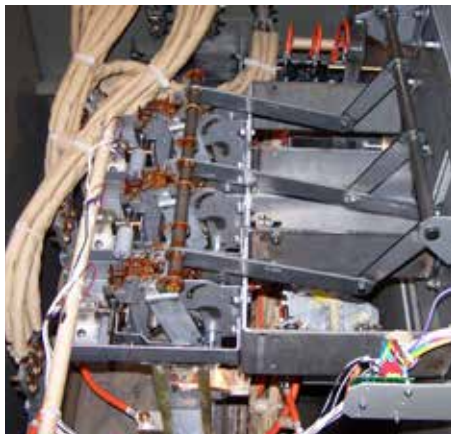
Figure 12. VFI—inside transformer tank.
