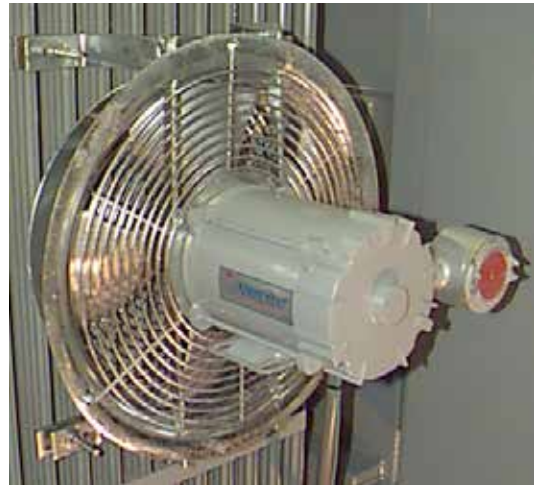
Figure 6. Transformer cooling fan.
