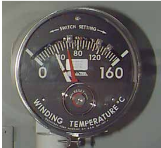
Figure 5. Winding temperature gauge.
