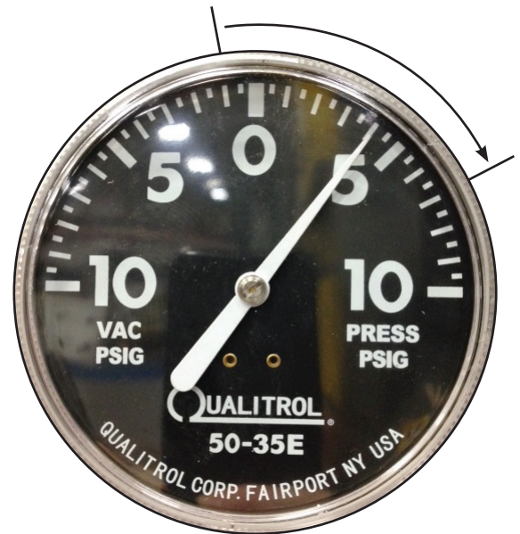
Figure 2. Acceptable Operating Range (-1 to +7 psig) for Transformer Pressure.
