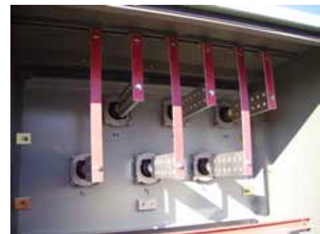
Figure 11. 12-pulse application with bushing supports.
