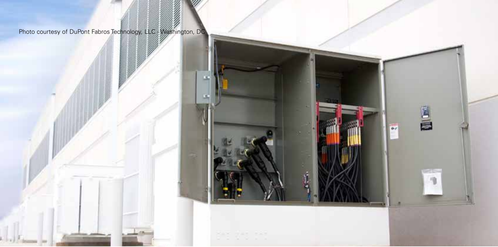
The top priority in data center operations is uninterrupted service. Shown here are pad-mounted Envirotran HDC transformers with a tamper-resistant cabinet for outdoor applications.
