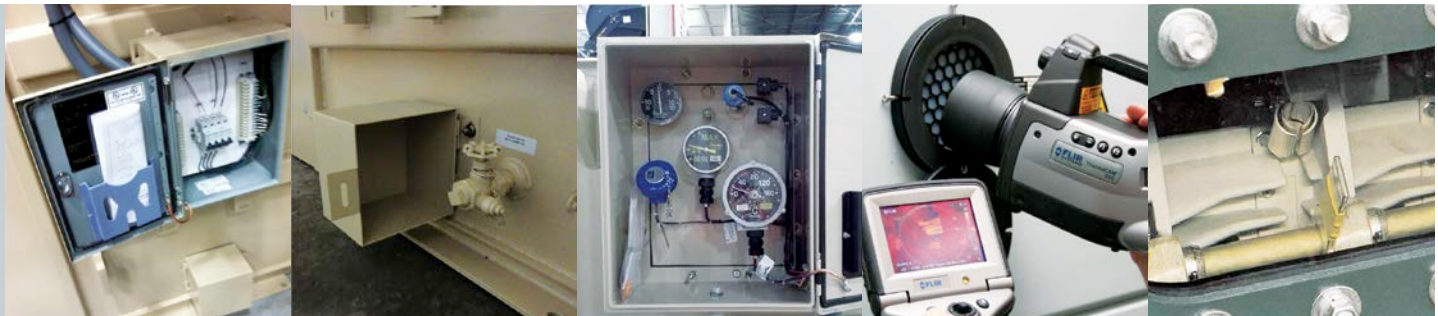
External control box
