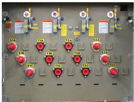
Figure 1. Compact single-sided units are available in vault and pad-mounted styles.
