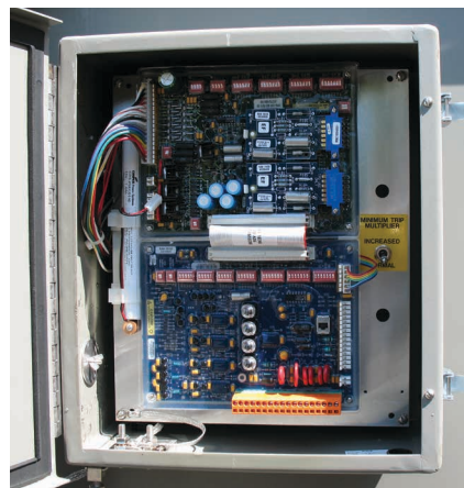
Figure 5. TPG control with SCADA shown.
