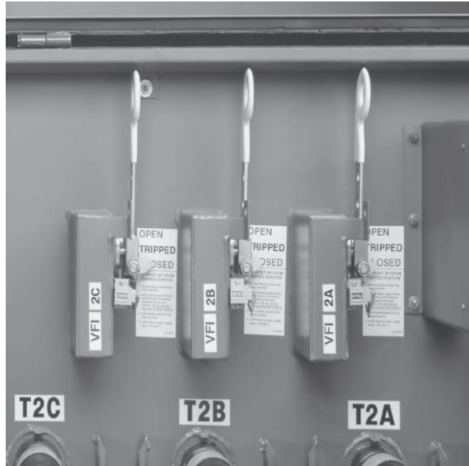
Figure 4. VFI switchgear operating handles, single-phase operation
