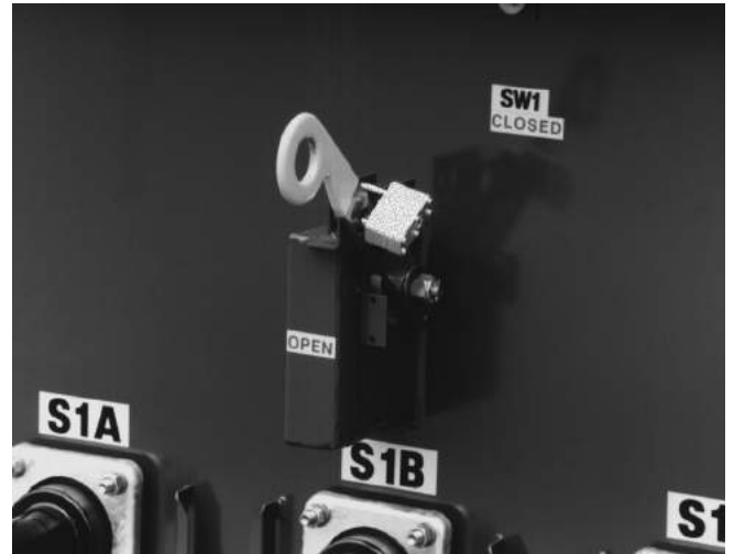
Figure 4. Switch operating handle shown padlocked in the open position
