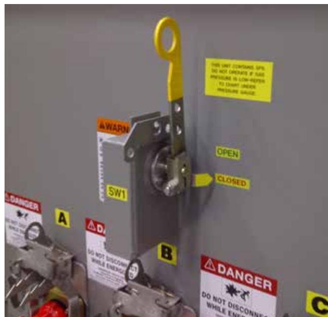
Figure 5. RVAC switch operating handle in the closed position.
