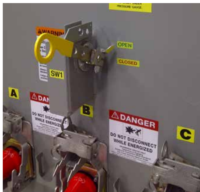
Figure 6. RVAC switch operating handle in the open position.
