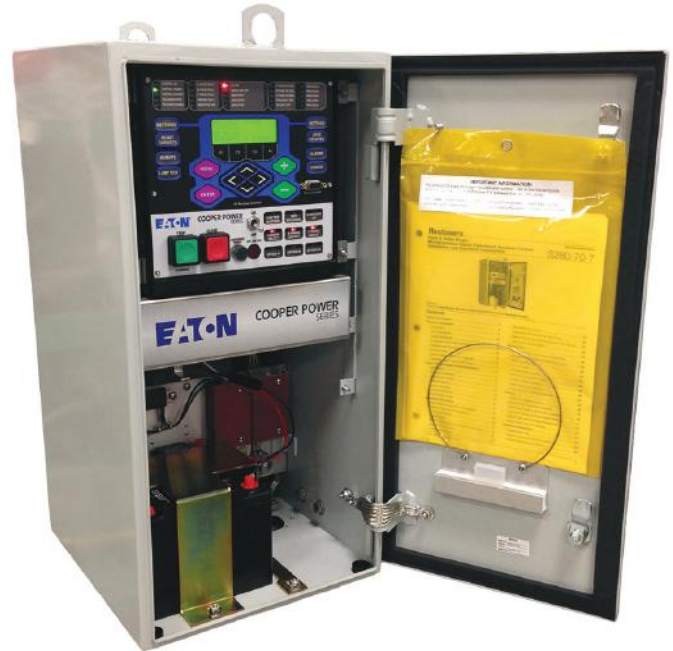
Figure 8. Recloser control cabinet - door open
