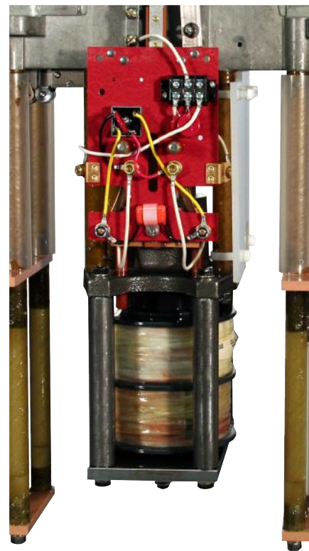
Figure 7. High-voltage closing solenoid contactor
