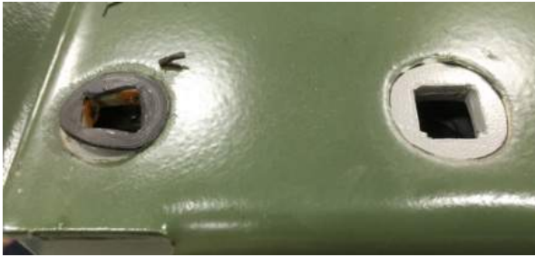
Figure 37. Typical condition of bolt hole area before cleaning. On the left, the bolt hole shows the bolt gasket adhered to the cover; on the right, the bolt gasket lifted off with the bolt when the bolt was removed.
