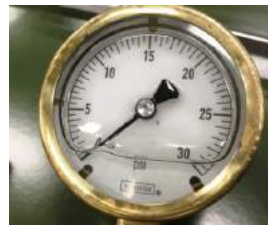
Figure 63. Close-up of pressure gauge
