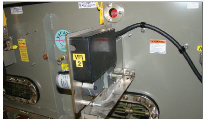
Figure 10. DC Motor actuator - limit switch enclosure
