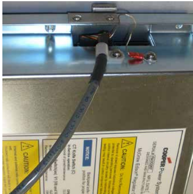
Figure 14. Connecting interface cable to CL-6A control panel.
