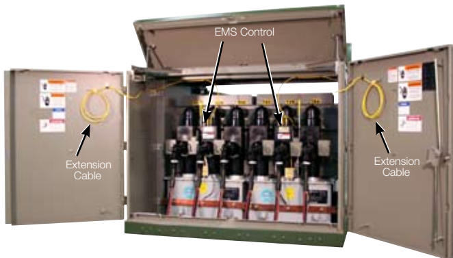
Figure 2. Edison Modular Switchgear/Control Cabinet.
