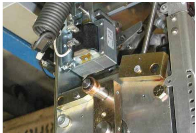
Figure 8. Spring hanging loose from housing.
