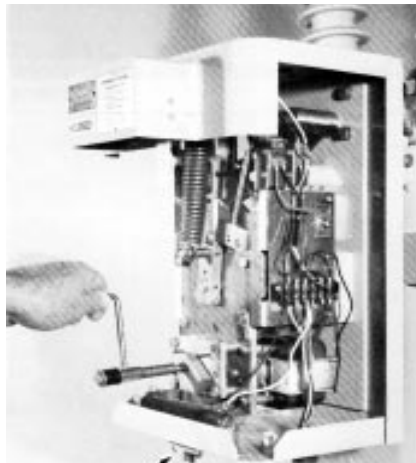
Figure 13. Manually cranking actuator to close switch.
