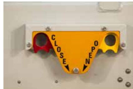
Figure 12. DAS switch manual open and close handles.
